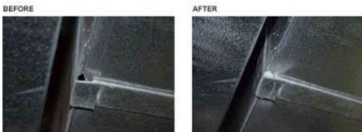
Sealing leaks from the inside: the aerosol sealant can fill holes as large as 5/8 of an inch across.
